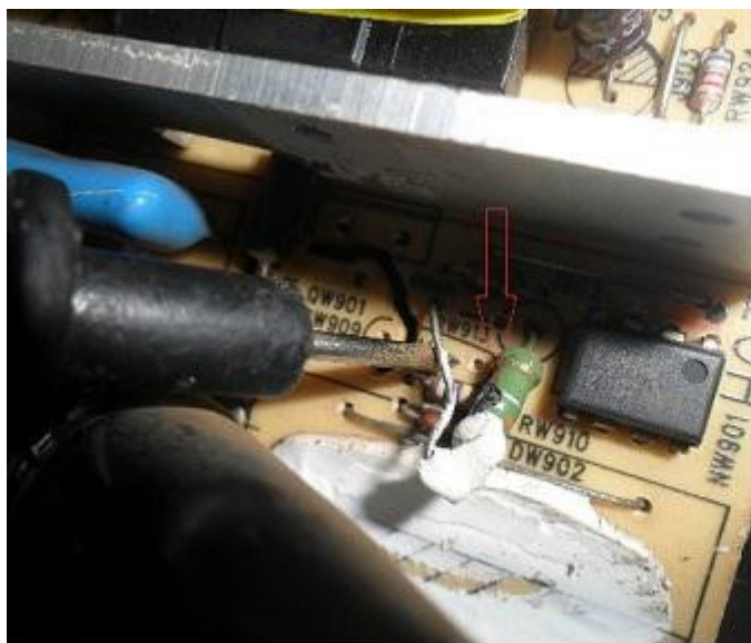
Fusabel Resistor Opened and Damaged.
